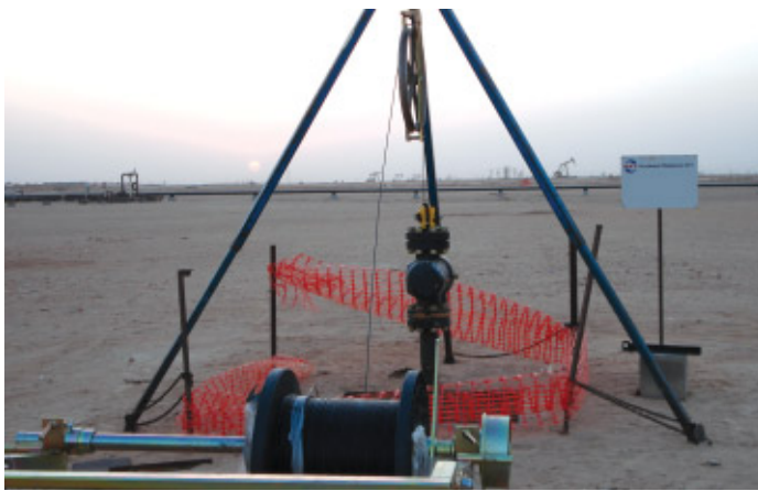
SensorNet FibreDip™ system in operation – spooling of self-supported sensing cable through the wellhead
